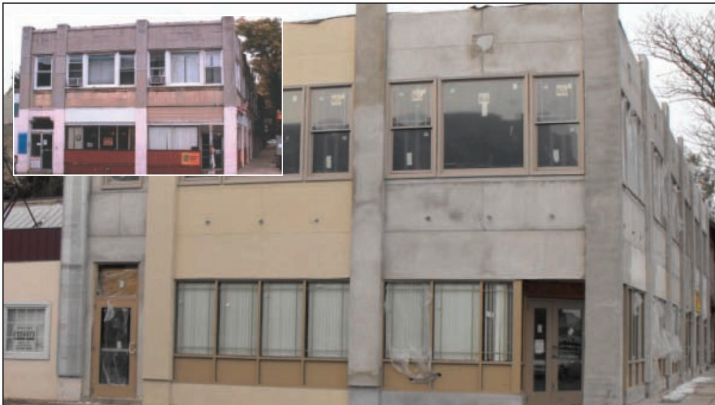
Before (inset) and in-progress improvements to properties at the corner of Lansdowne and Baltimore Avenues.
